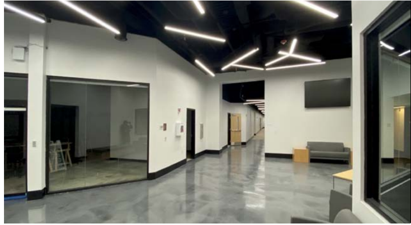
Harbor Hall, at USF St. Petersburg campus, in the process of renovation. Opposite page: Ribbon-cutting of the new Generator space in St. Petersburg.
