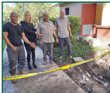
Dante Fields, VP Carole Post, Clint Franklin, and Terry Pilon next to the fixed pipe.
