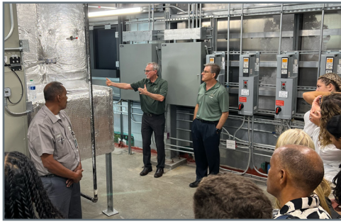
Don Crosby showcasing the Honors College DOAS-1 (Dedicated Outdoor Air System), which is used to reduce the building's energy consumption.
